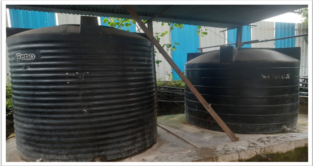
Drinking Water Tank at labour camp
