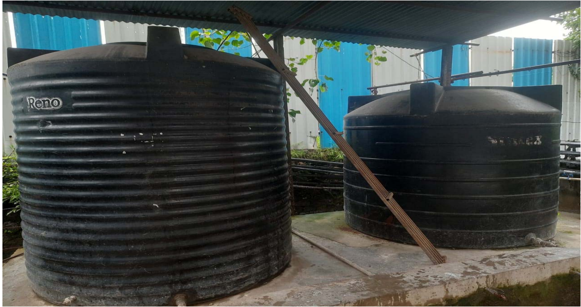
Drinking Water Tank at labour camp
